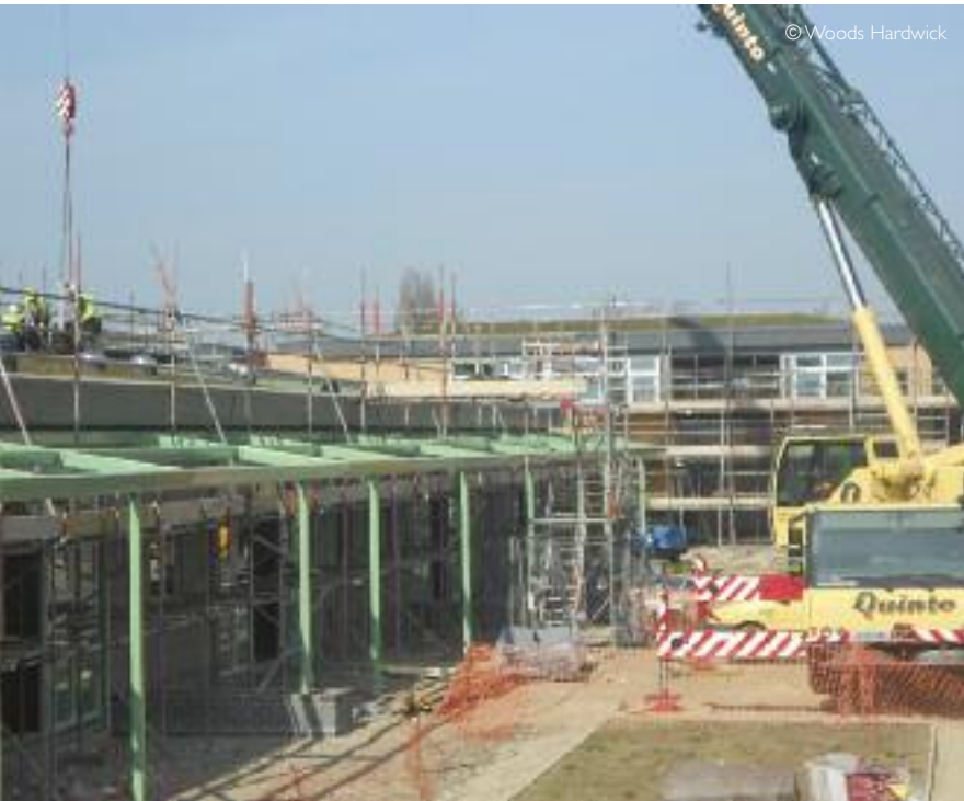
The school while under construction; opposite showing the main 'street' runs through the school with classrooms off it
